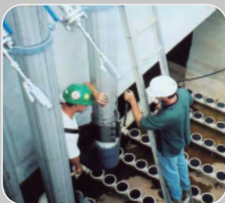
▶ Canada : water purification facility
