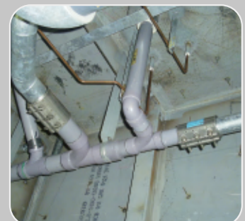
▶ PVC+Steel Pipe Connection
