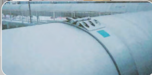
▶ 48 "(1,200A) MF-RL Canadian power plant cooling line
